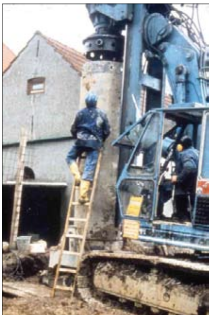
Screwing and fastening the column casing to the driver using a ladder
